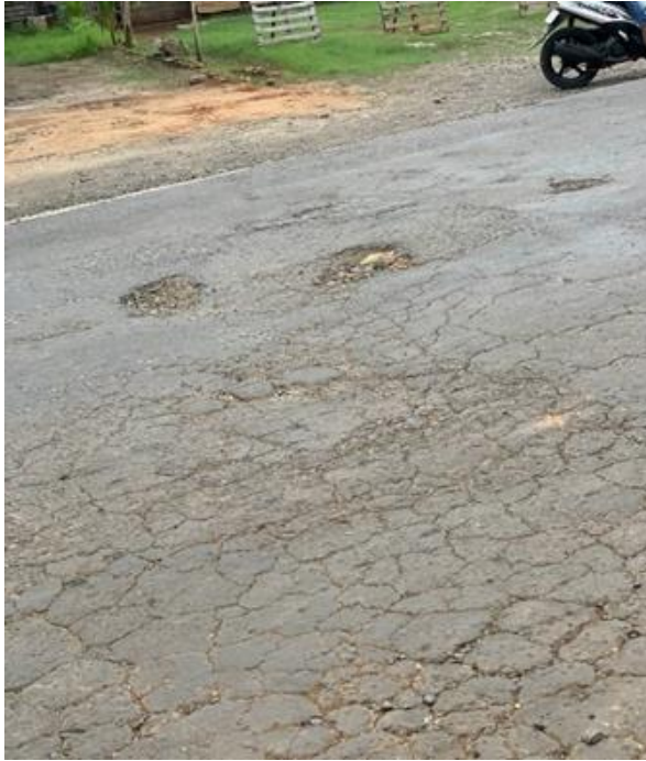
Figure 3. Potentially road cracking
