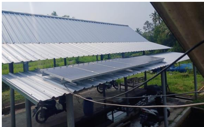
Gambar 3. Panel surya terpasang
