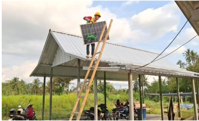
Gambar 2. Instalasi Panel Surya
