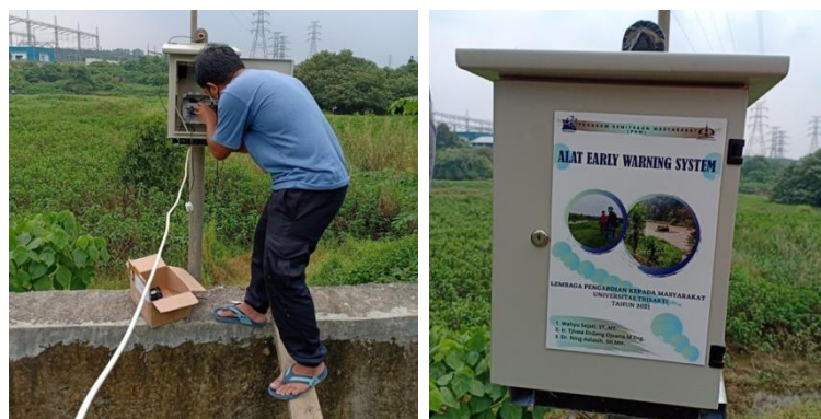
Gambar 3. Pemasangan alat early warning system (EWS)
